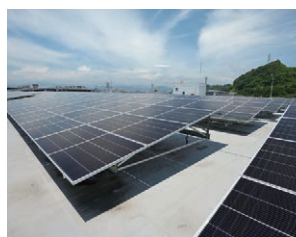
Hiroshima Plant (Head Office) building with solar panels installed on the rooftop
